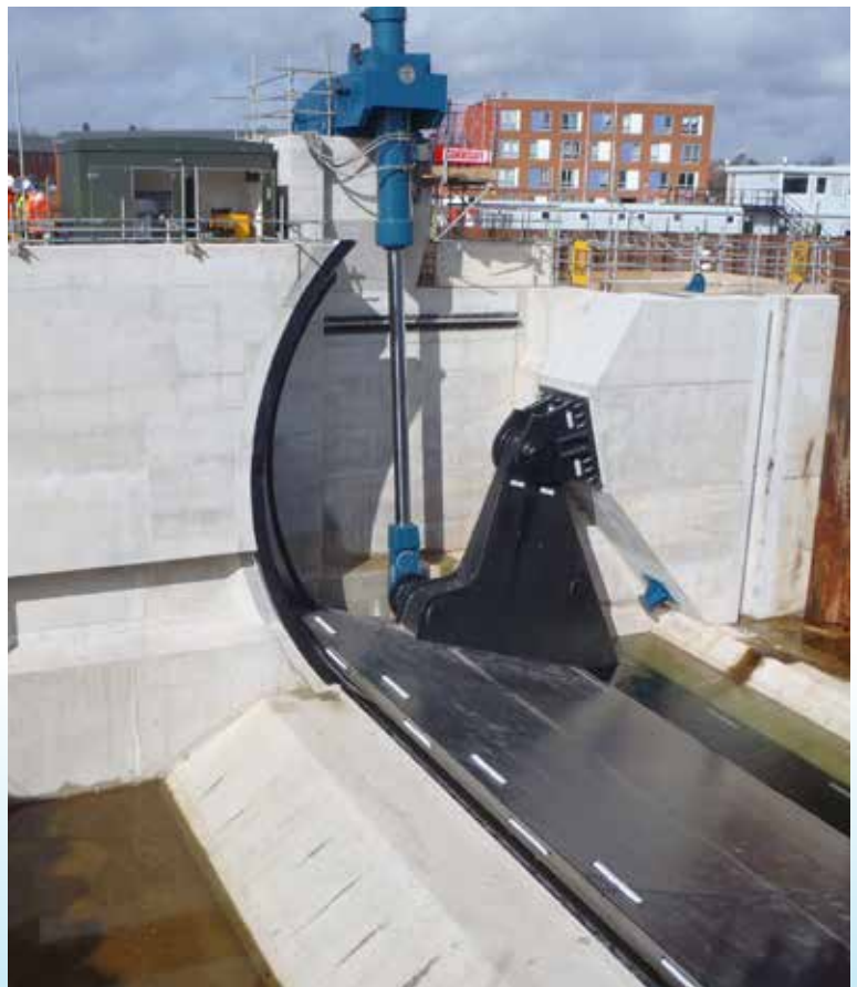
Ipswich Barrier dry commissioning (gate lowered)
