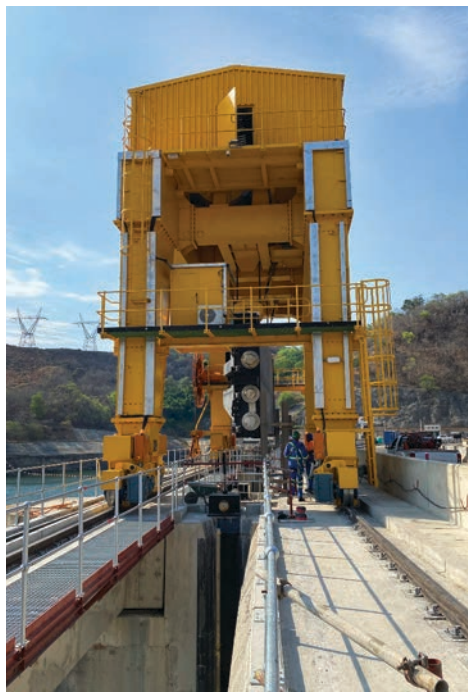
The Kariba Dam 510 tonne gantry crane, designed and fabricated by Morris Material Handling in South Africa.
