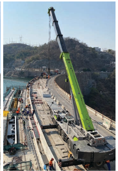
View towards Zambia - sluices 6, 5 and 4 are visible. Sluice 4 has a section of emergency gate stored, sluice 5 has the stop beam grapple stored, sluice 6 is empty. The 250 tonne mobile crane, supplied as part of the Spillway Rehabilitation Project, assisted in the final stages of the works.
