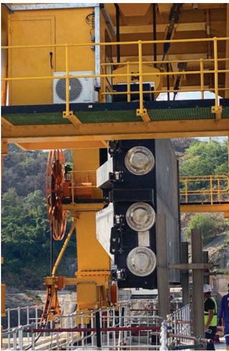
Two of the six sections of the emergency gate hang from the 510 tonne gantry crane. This gate comprises six sections that are assembled by the gantry crane in any one of the six spillway sluices. The gate is designed to close in unbalanced conditions against a flow of up to 1,500m 3 /s.
