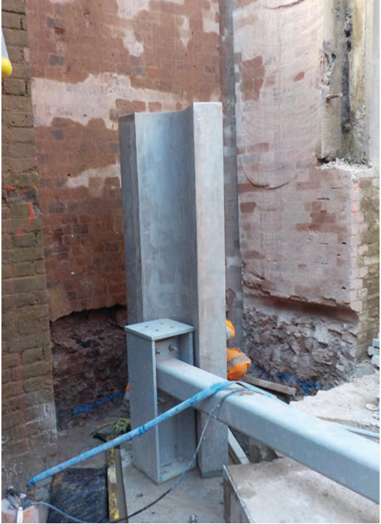
Pintle base plate and quoin section, with positioning jig installed to ensure correct tolerances are achieved
